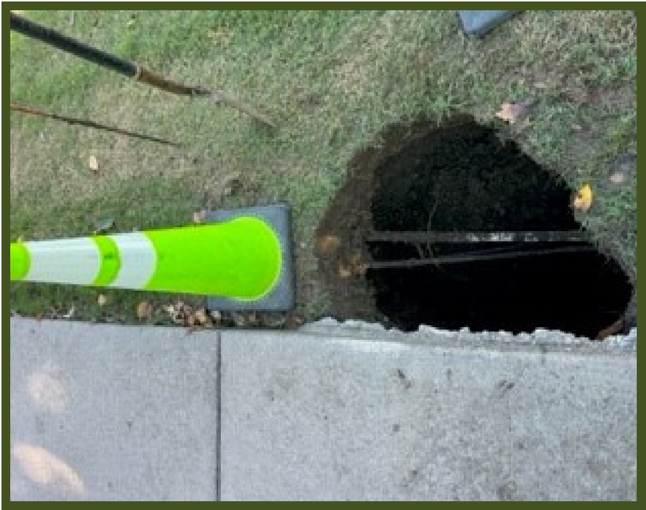
EMERALD BAY SINK HOLE REPAIR BEFORE
