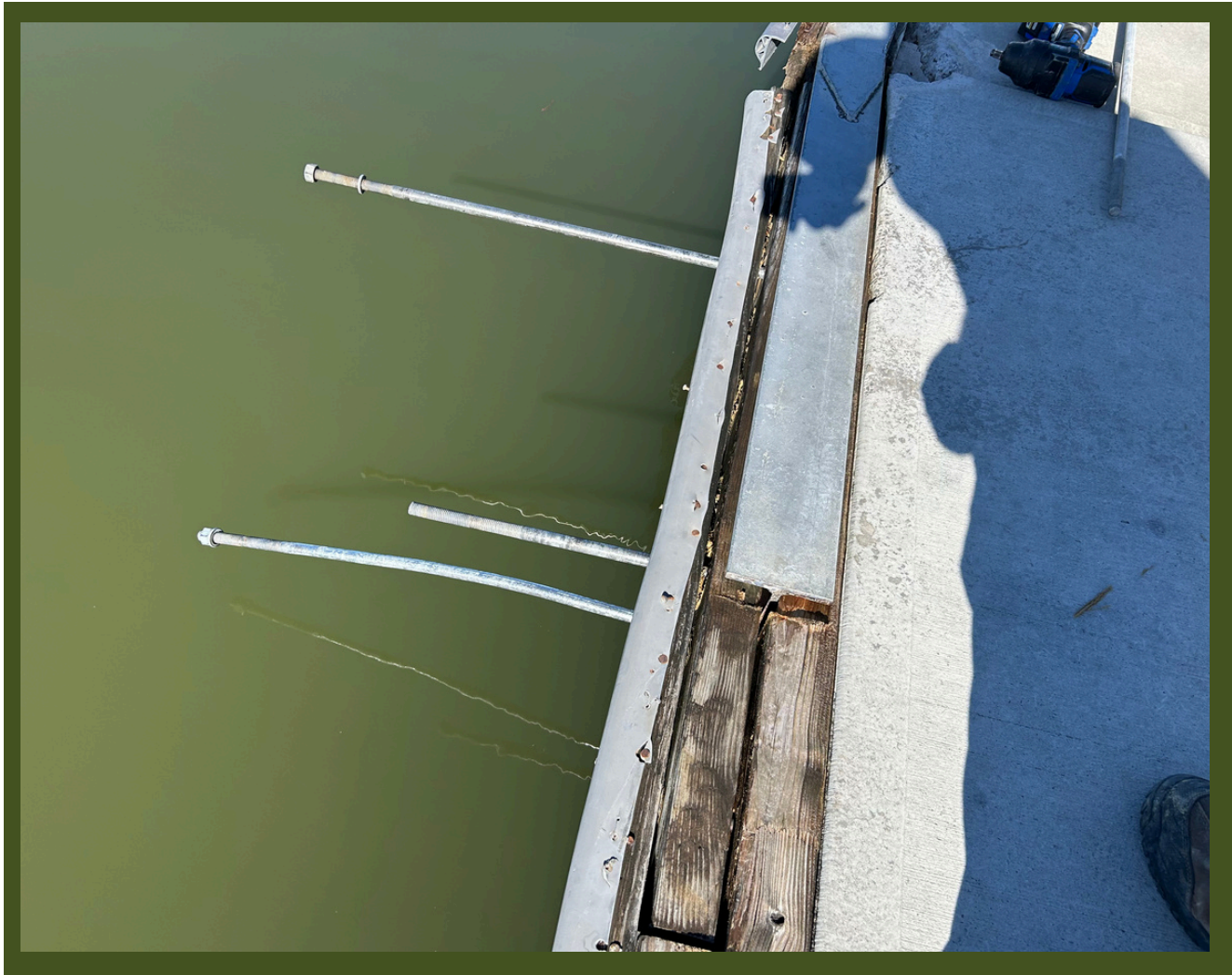
THE HARBOR BOAT DOCK DAMAGE
